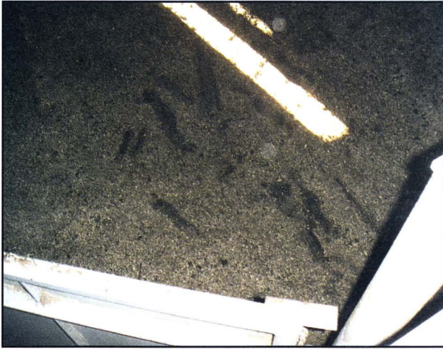
Photo 7. Worn cement results in slips on the dock.
