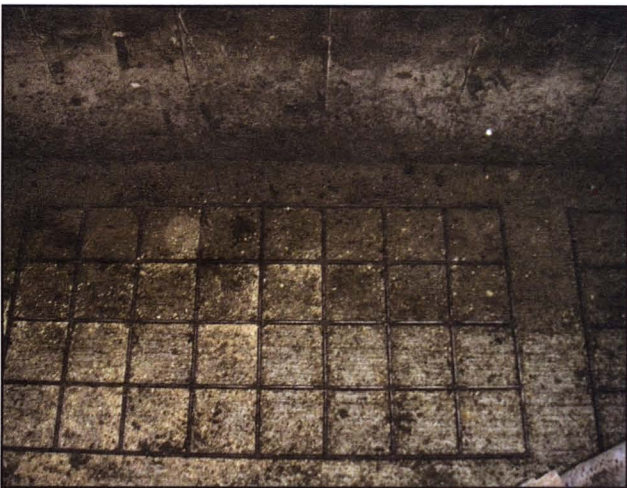
Photo 13. Hinged floor grating lifts for cleaning.
