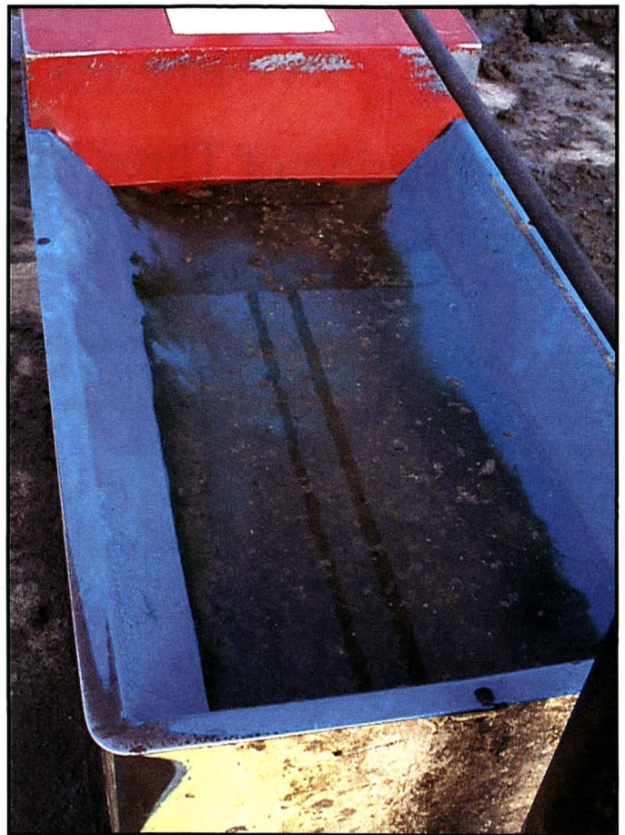
Figure 1. Water tank prior to cleaning.
