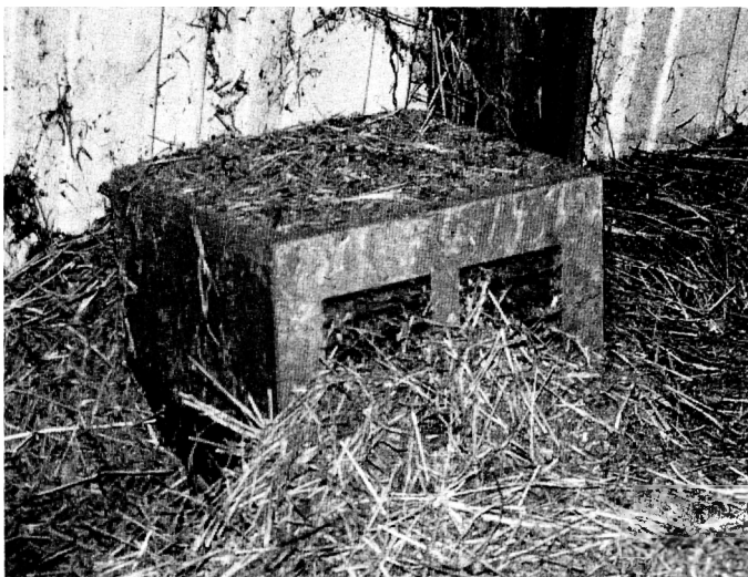
Figure 14. Air supply to ceiling intake in stable below must enter through this plugged opening in mow of two-story barn. Little air can pass through. Results, poor ventilation system performance.
