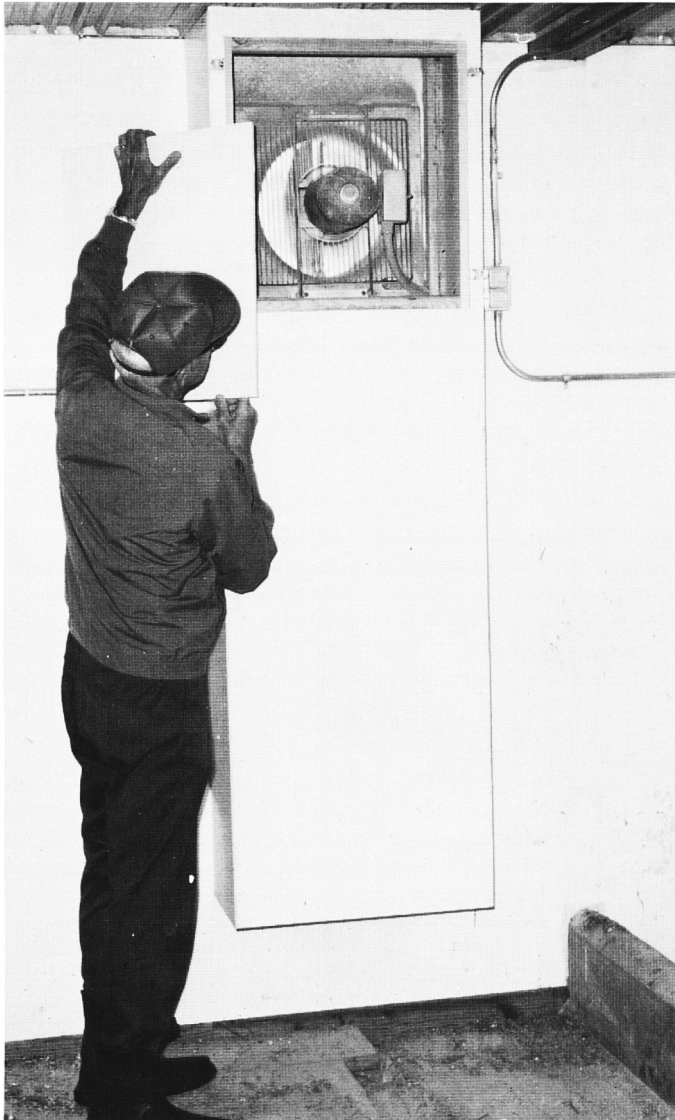
Figure 8. In winter, air near the floor in a livestock building can be as much as 10 degrees cooler than air near the ceiling. To conserve heat and energy, a duct as shown should always be used around the continuously operating exhaust fan or fans. An equal amount of moisture but less heat is removed than when air is exhausted from the ceiling, making a higher ventilation rate and thus greater dilution of contaminated barn air possible.
