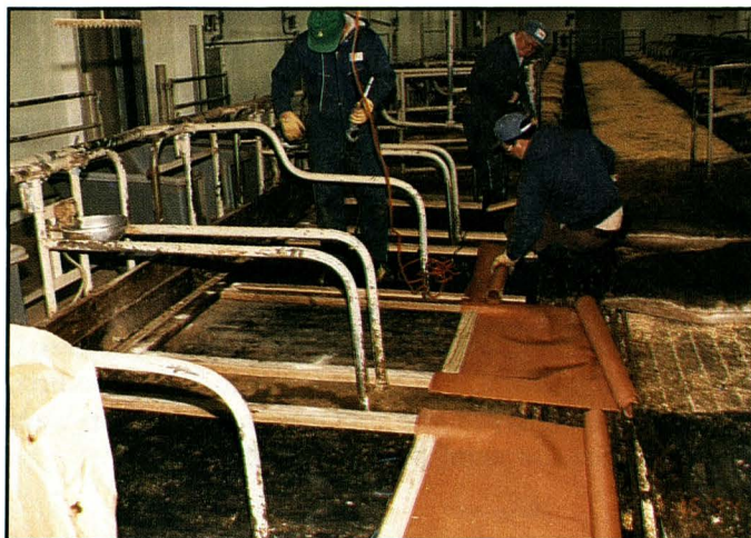
Figure 4. Construction of type 2 and type 3 mattresses showing: A) placement of 2 x 4 inch treated lumber around the tie stall, B) the shredded rubber fill, and C) securing of each mattress to the tie stall.
