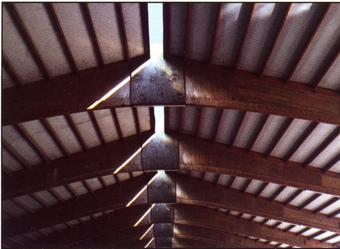
Figure 2b. Image of roof ventilation for confinement facility used in study.
